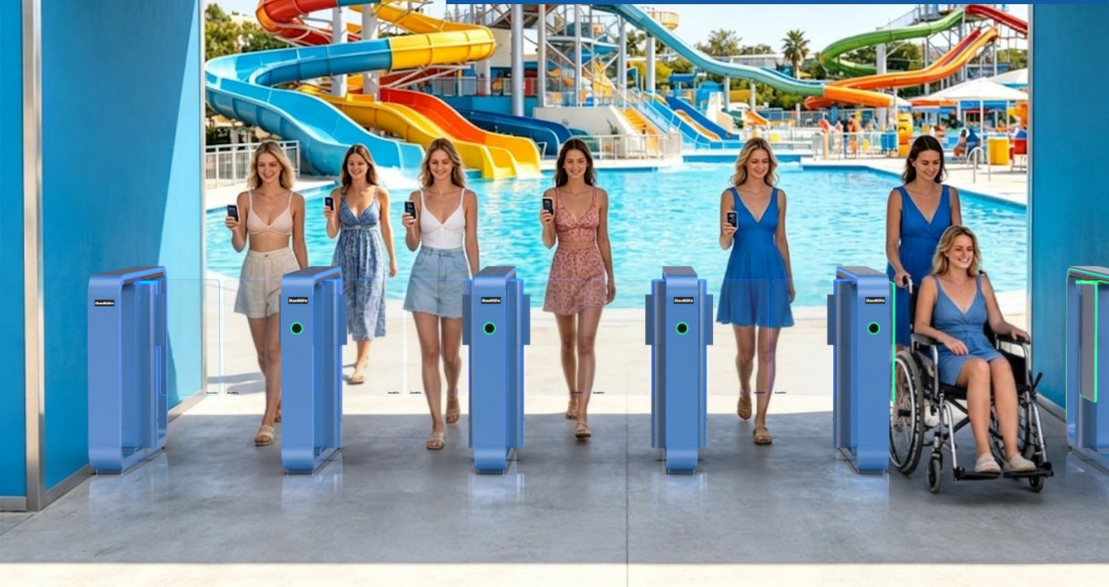
Five lanes with a disabled lane installed at the water park entrance.
